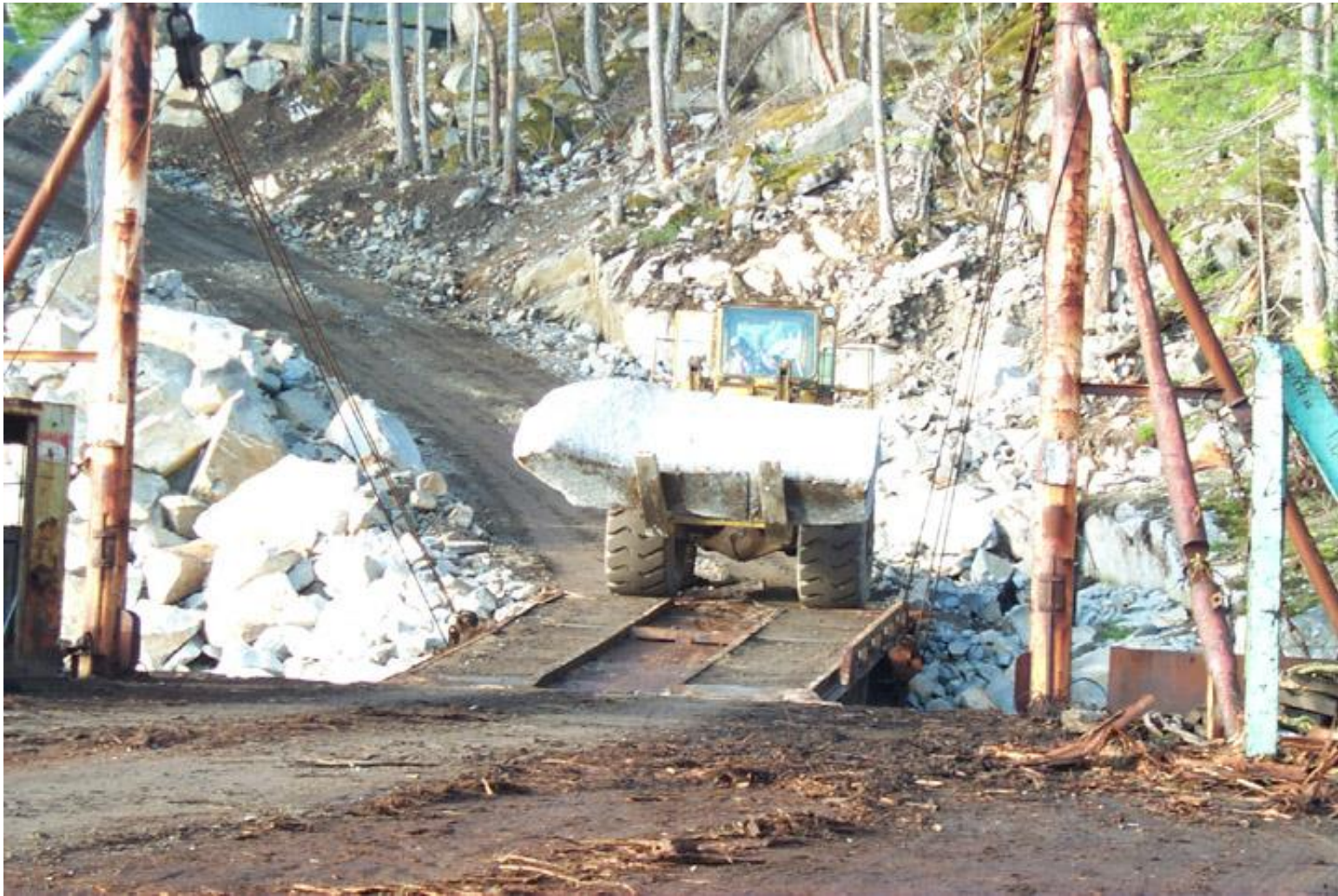
A front end loader hauls the granite blocks to a barge in Jervis Inlet..
