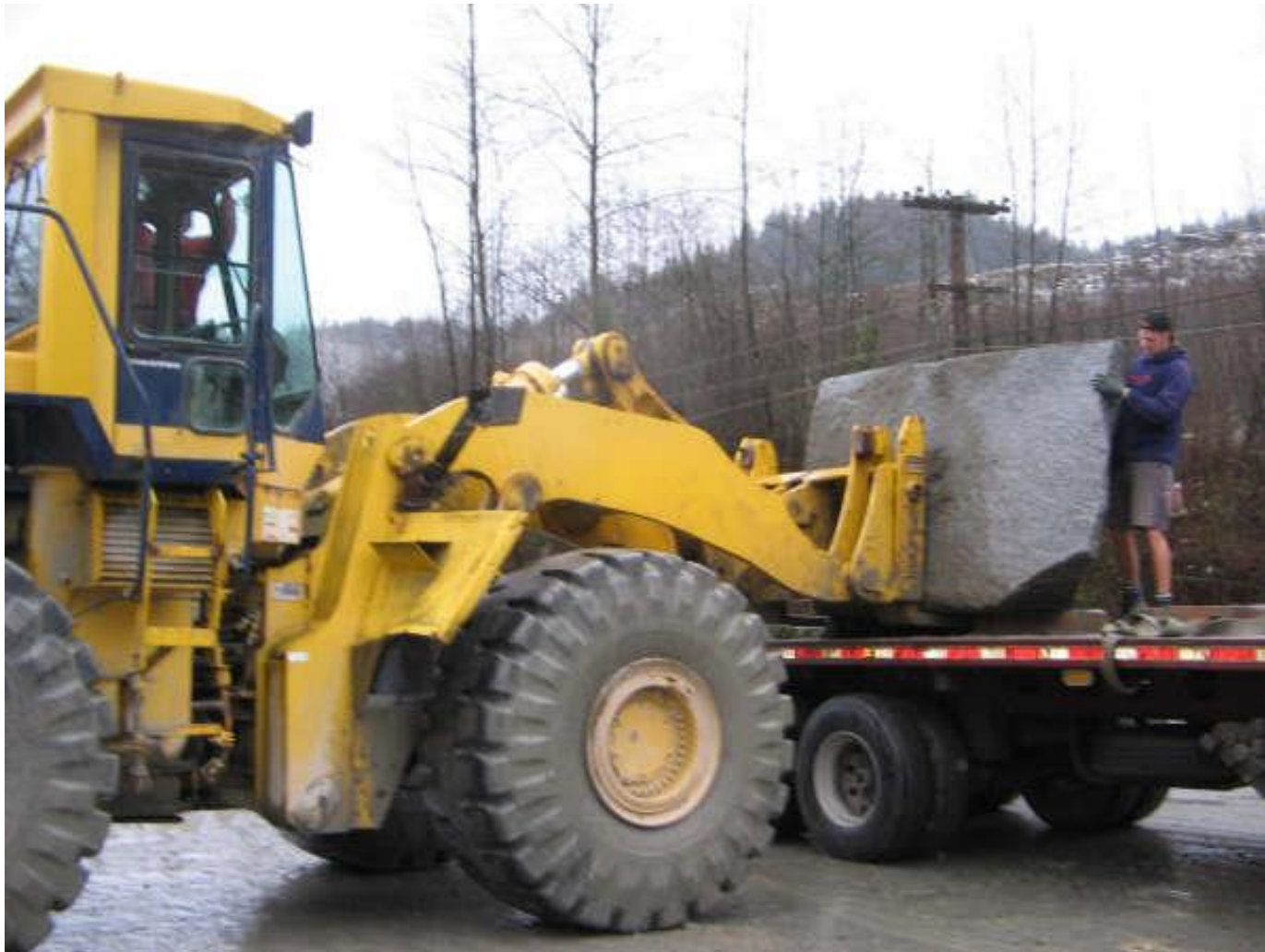
Offloading the granite blocks with a front end loader onto a flatbed truck.
