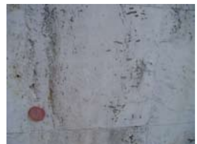
Figure 26 – Travertine wall panels showing irregular lamination and scattered to sub-parallel vugs; Transport Canada building.
