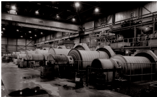
Rod and ball mills within the concentrator facility of Gibraltar Mine, where fine ore is ground further before being passes on the flotation unit.
